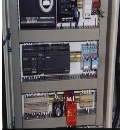
Power Panel for Parts Elevator
